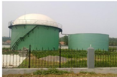
Babak Ternak Sapi Chengdu Tank Top Gas Holder Volume: 250m 3
