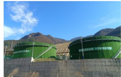
Tangki air darurat kebakaran Volume: \phi 27m^2 , \phi 31m^2 \phi 12m^1 , \phi 10m^3
